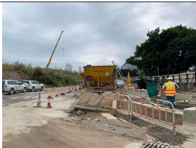
Q6: Wastewater treatment facility 24 cu. m.
