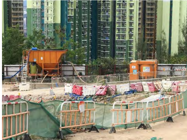
Q1. Wastewater treatment facility 30 cu.m Sedimentation Tank + AquaSed of 15 cu.m per hour + WETSEP
