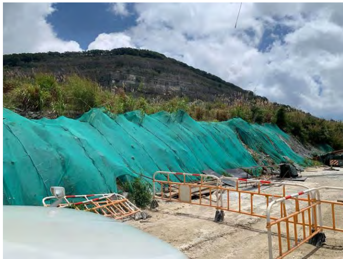
Impermeable cover for slope at System A.
