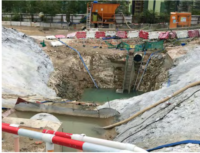
Paving for exposed slope to reduce dust dispersion & mitigate the silty runoff generation at Q1.
