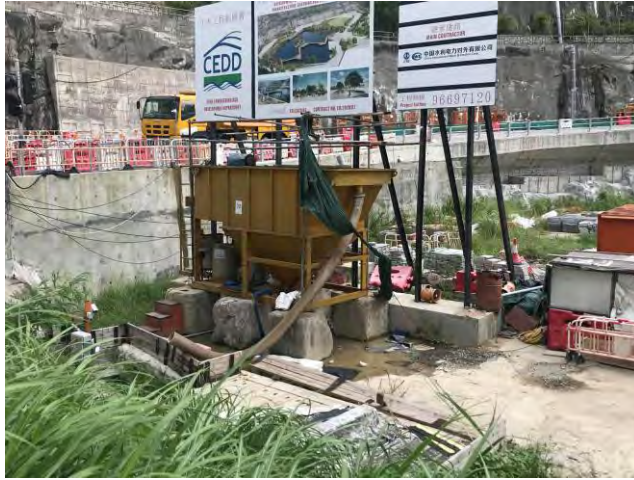
Q7. Wastewater treatment facility 30 cu.m Sedimentation Tank + AquaSed of 60 cu.m per hour
